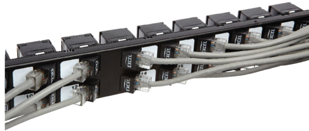
D. Keystone Jacks mounted in chrome style patch panel
